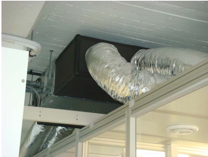
Image 20: 5kW air conditioning system
