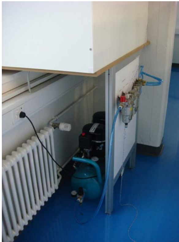
Image 10: Compressor to generate compressed air
